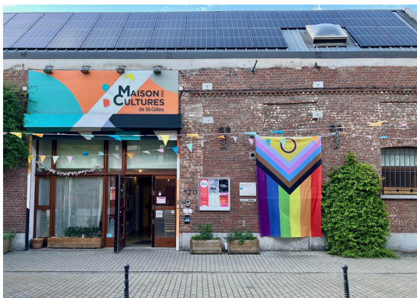
Photovoltaic installation on the roofs of the Maison des Cultures in Saint-Gilles
